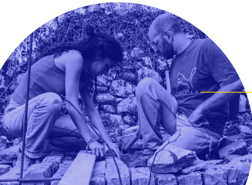
Two participants during a hands-on workshop on traditional building techniques 'KalderimiX2' (Photo credit: Athena Apostolou | Blk © 2019)
